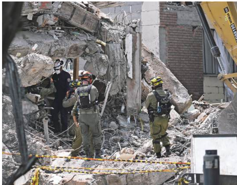
Israeli rescue workers search amid the rubble of the fallen Vanessa building in Cali, Colombia, yesterday, eight days after a 7.4 earthquake. – AFP
