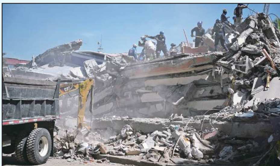
Rescue workers help remove debris in search of survivors in Cali, Colombia, yesterday, three days after the country's 7.4-magnitude earthquake. The confirmed death toll from the temblor that struck western Colombia on Monday has risen to 265, with over 3,500 individuals injured and nearly 500 officially listed as missing. — AFP
