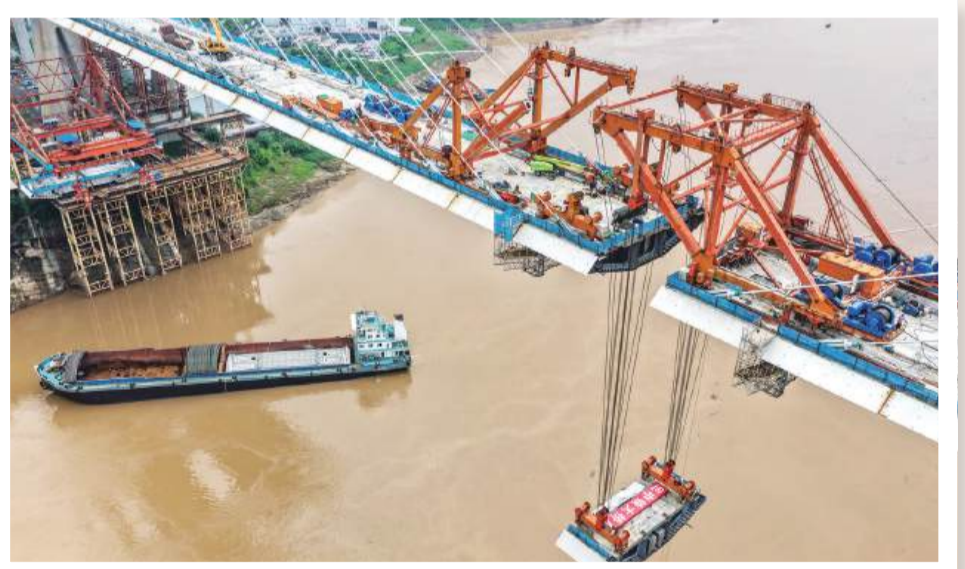
This aerial drone photo taken on Tuesday shows the construction site of the Shituo Yangtze River Bridge along the Chongqing-Wanzhou High-Speed Railway in Chongqing. The deck of the railway line of the Shituo Yangtze River Bridge successfully completed its closure yesterday. The bridge has a total length of 1,416.9 meters, with the main bridge spanning 1,056 meters. The deck of the highway lanes is scheduled to be closed by the end of this year. – Xinhua
