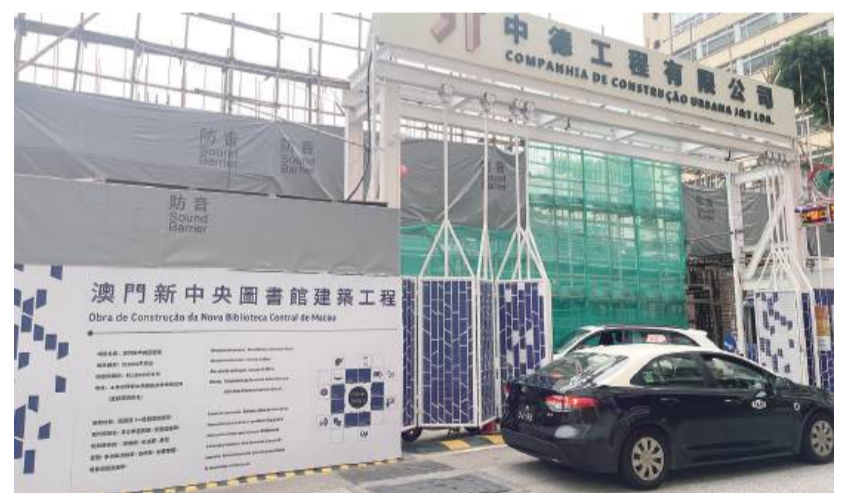
A taxi is driven past the construction site of the ongoing new central library project on Avenida de Sidónio Pais yesterday. — Photo: Armindo Neves
